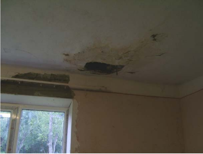
Leaking roof in classroom
